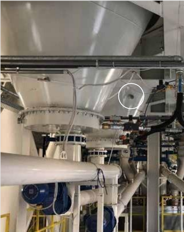
VBS (aireadores) - Silos
